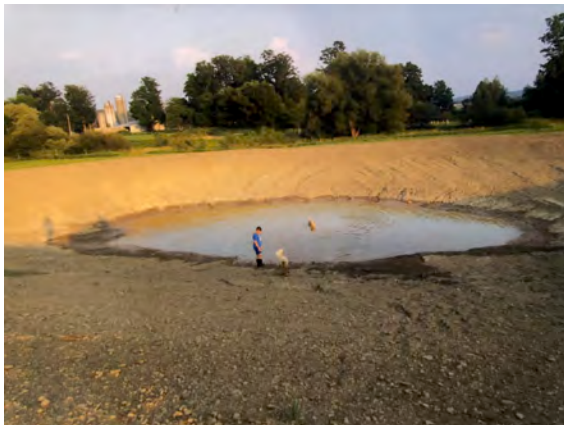
Nicholas, Daisy and Duke checking out the newly constructed retainer pond to manage run off.
